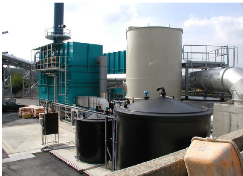
Figure 2 RTO-plant of MBA Singhofen, acid scrubber at front
